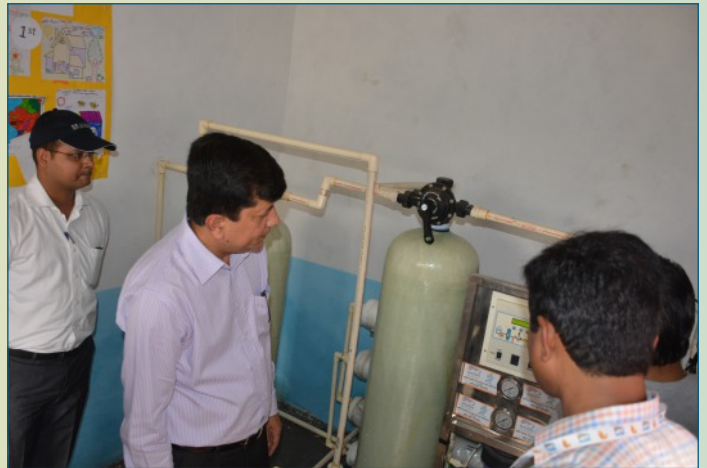
RO drinking water facility
